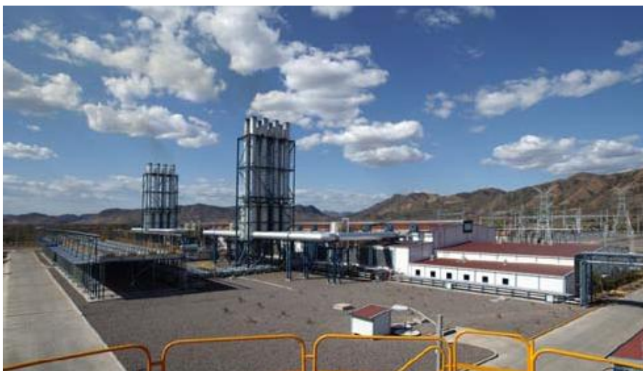
The Lufussa Pavana III base load power plant is located in Honduras and consists of 16 Wärtsilä 18V46 engines having a total output of 273 MWe.
